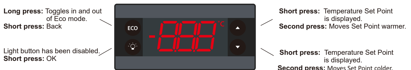
Figure 5: Fascia of the control panel
